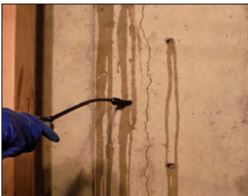
3. Flushing crack with water to ensure sufficient moisture is present for grout to properly react.
